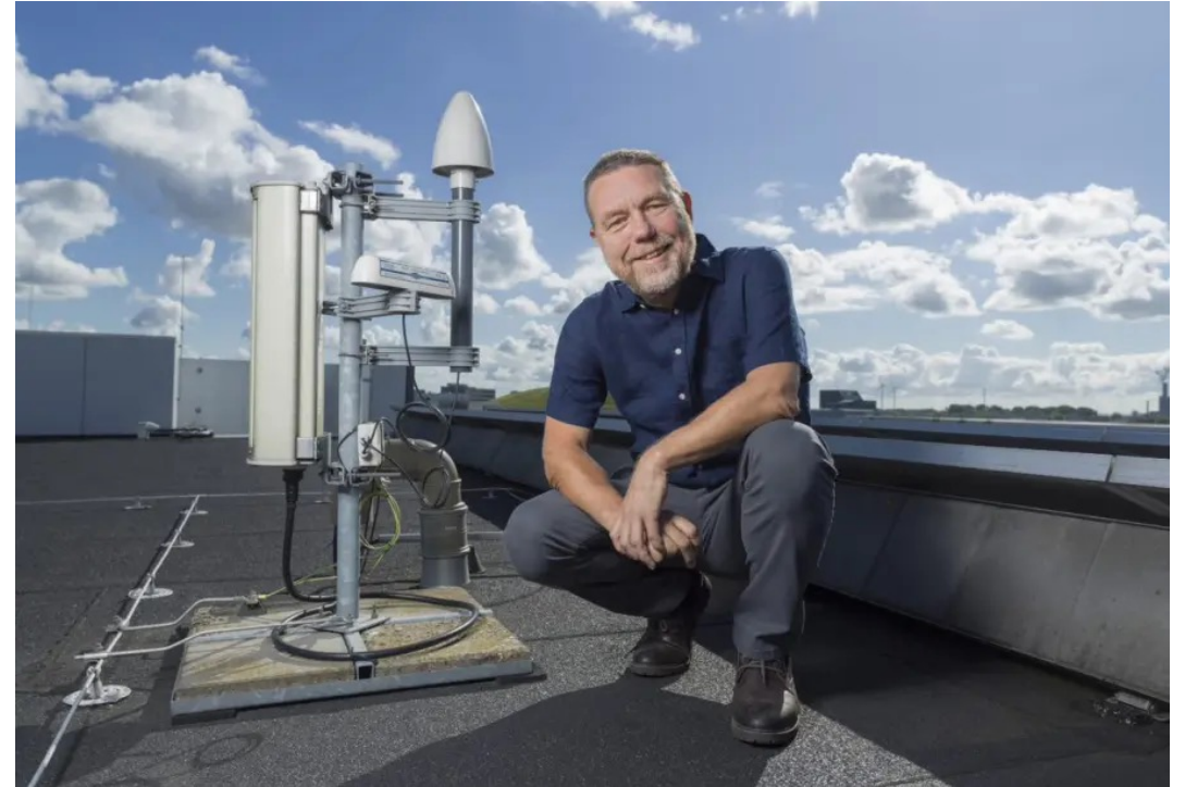
GPS/Galileo and DCF77 antennas on the roof of the SIDN building
