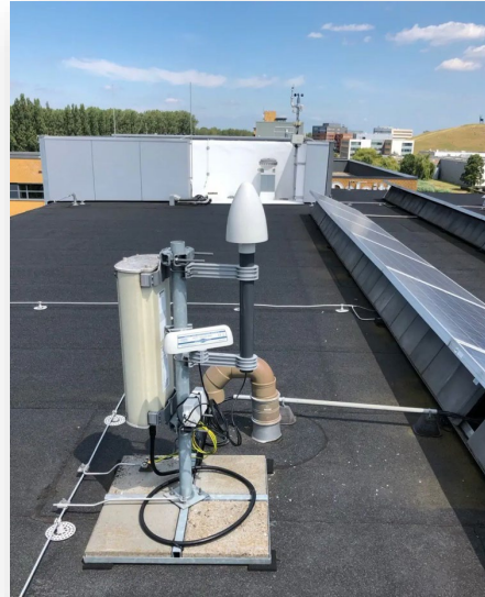
Provide well-managed and secure time services
